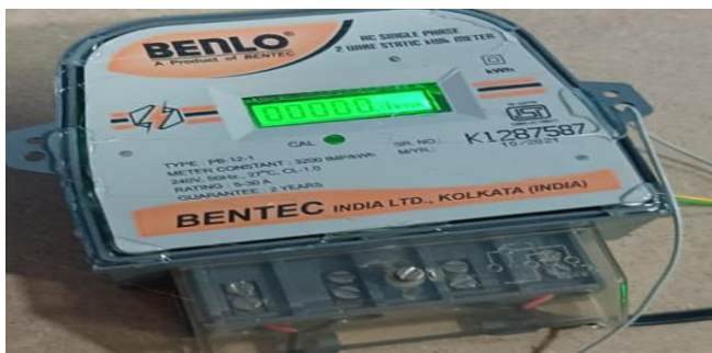
Fig.13: Energy meter reading showing in transmitter section
