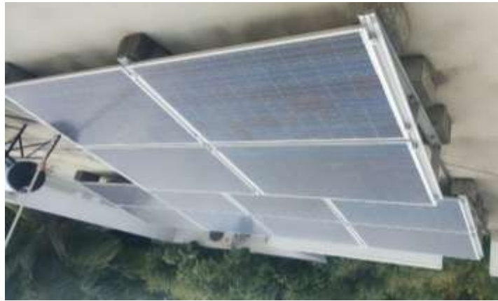
Fig.15.Rooftop Real Time Solar panel Arrangement
