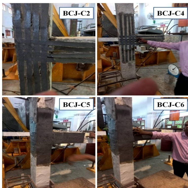
Figure 7(c) Crack patterns of 30% axially loaded CFRP retrofitted specimens
