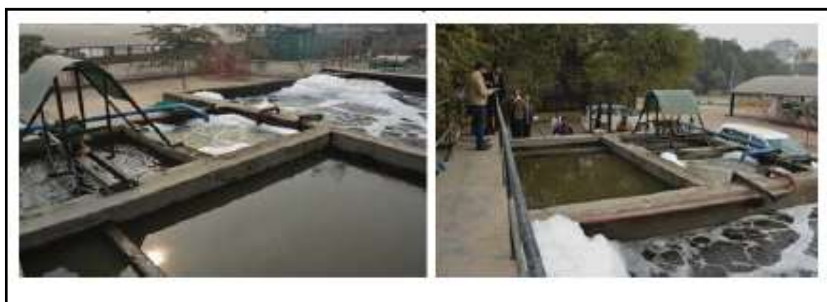
Figure 9: Chemical liquid waste: Separate collection system to STP-AIIMS
